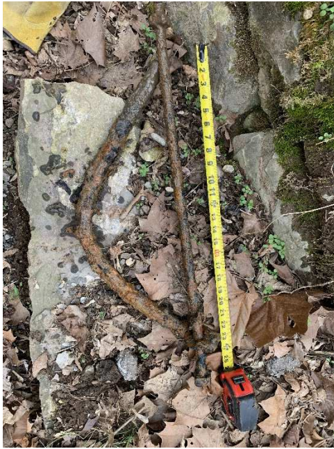
Figure 15 – Iron bars found at the bottom of the wall
