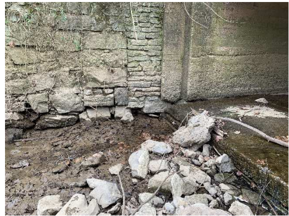
Figure 17 - Slab at the base of the bridge was placed on timbers. There is a slot or notch in the concrete abutment, likely used to slide in boards to dam the water during repairs to the turbine.
