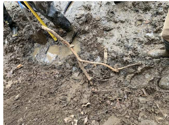
Figure 8 - The sediment above the timbers was excavated by DPW personnel and can be seen in the photo.
