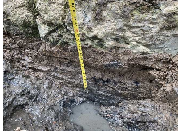
Figure 11 - An 8x8 inch timber was seen to run parallel to the wall under its face. End of the tape measure is in contact with the timber.
