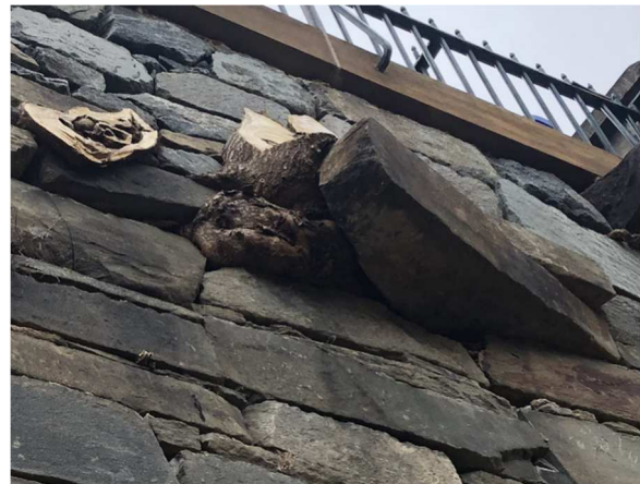
Figure 20 - Example of wall damage by vegetation, This stone was pushed out of the plane of the wall by the growth of tree roots (located at the C&O Canal in Washington DC)
