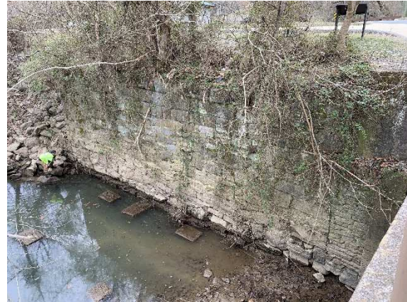
Figure 16 - Foundation wall for the Mill. The stones in the tail race were likely foundation stones for the turbine.
