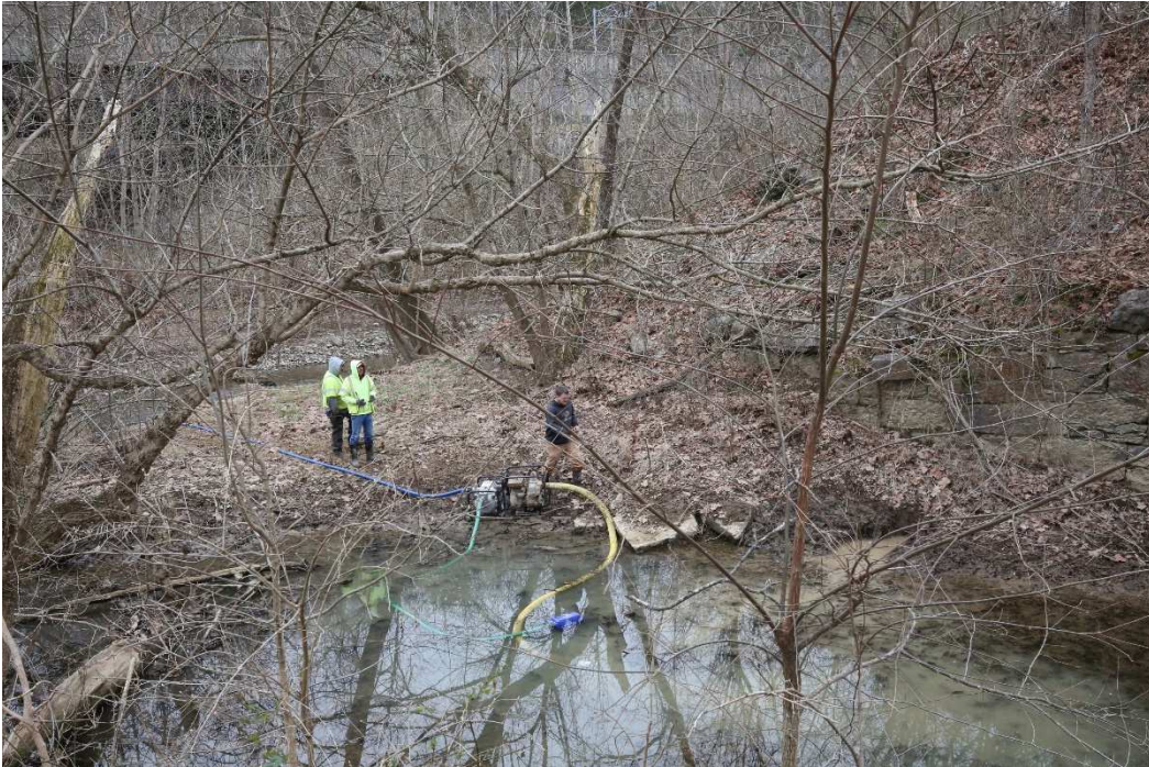
Photograph 1: Workmen using pump to dewater the site. The stone wall is visible on the right.
