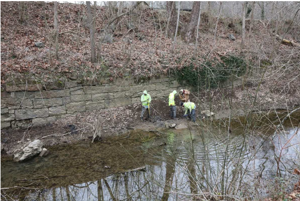
Photograph 2: Workmen digging access hole to timber. Stone wall is visible behind workmen.
