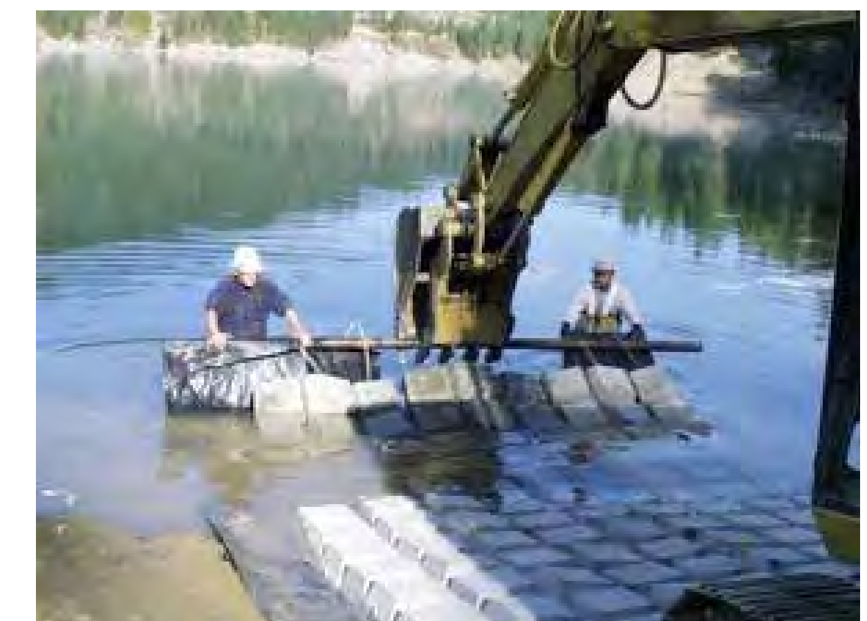
O. Fishing access point - image showing articulated concrete blocks (ACBs) that could be used as a stabilized fishing access area where shore gradients are low
