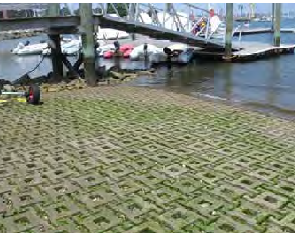
A. Canoe Launch - image showing articulated concrete blocks (ACBs) that could be used to reinforce the canoe launch
