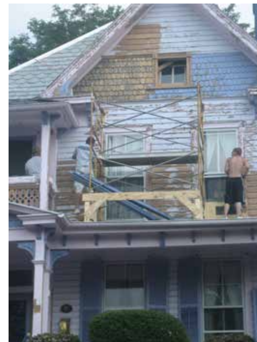
Properly prepared wood siding, shingles, & detailed trim is absolutely essential to a quality paint job as shown on this Queen Anne-style residence.
