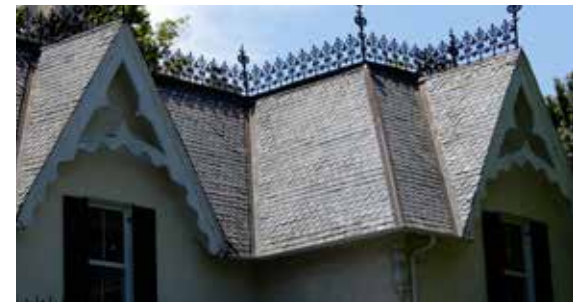
Metal cresting is found on a number of historic houses in the districts.
