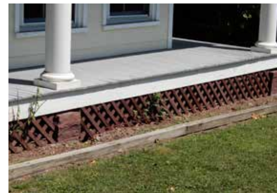
Porches sit on foundations that are typically masonry piers with some type of lattice filling the space between the piers & enclosing the space under the porch.
