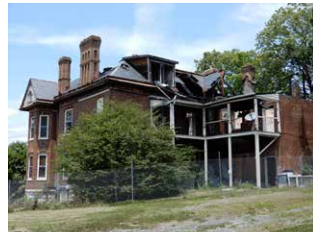
This historic house, damaged by fire, would benefit from the removal of burned materials and adding temporary materials and venting to better preserve the remaining historic fabric if the dwelling is not going to be demolished.
