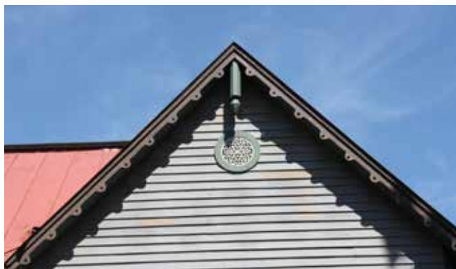
The gable of this dwelling is trimmed with a decorative wood bargeboard along with a circular vent.
