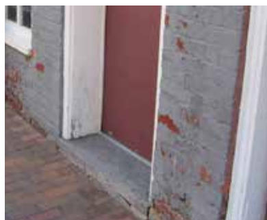
Rising damp from the ground below can saturate bricks & cause paint failure.
