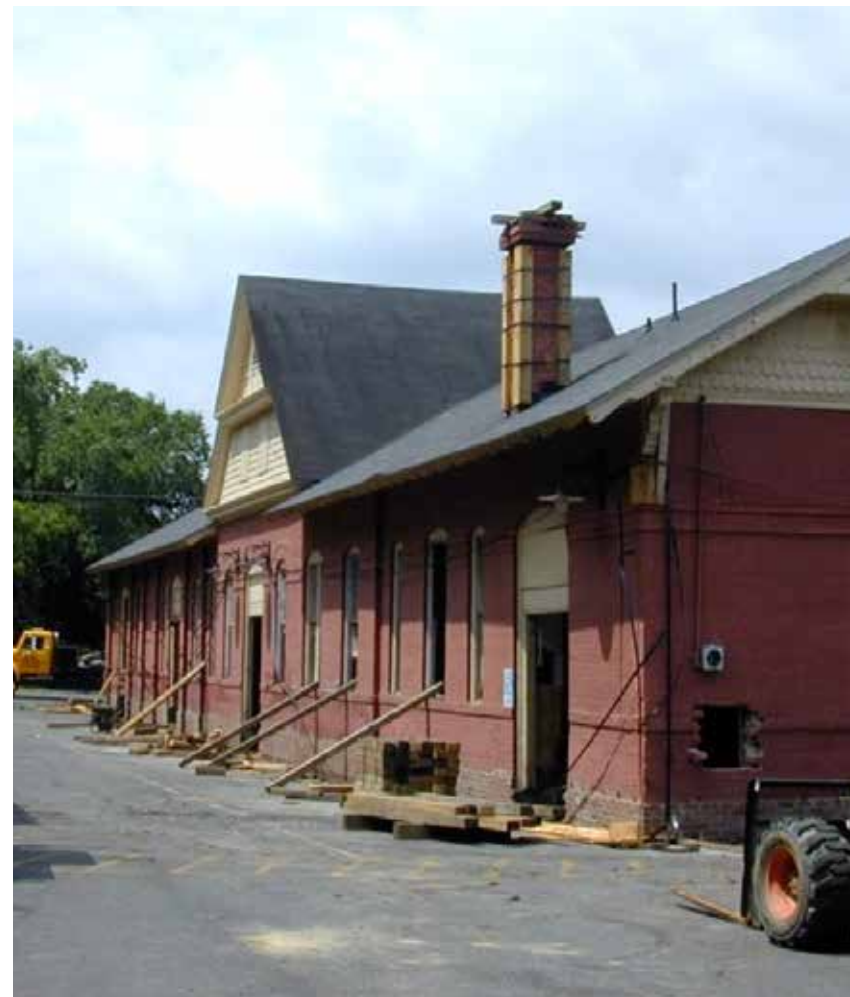
The train station in Lexington, VA was carefully relocated to allow for new construction on the campus of Washington & Lee University.
