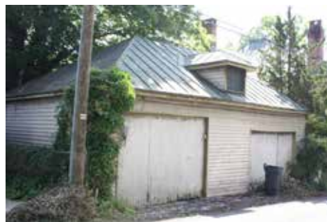
This older outbuilding has historic elements and materials such as the standing-seam metal roof, the dormer and original wood siding.
