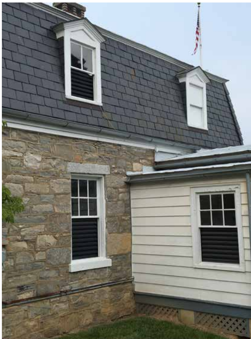
This historic house has been mothballed using vents in the windows to provide air circulation & prevent moisture & mold.
