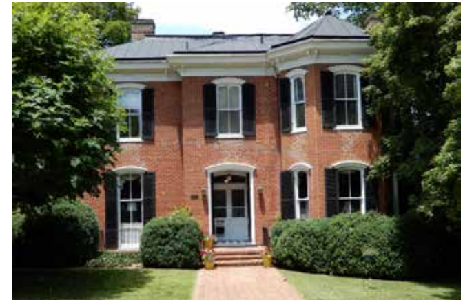
This Italianate styled dwelling has a prominent projecting bay and arched openings. Its original porch is likely missing.
