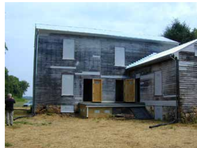
The mothballing of this historic house included enclosing openings with plywood for security purposes. The windows' plywood panels included vents to allow for ventilation.
