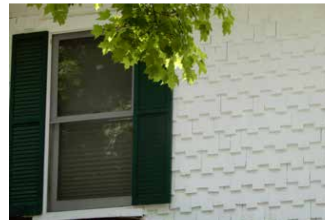
Wood shingles are used throughout the district on a variety of building types and styles. Here the shingles are installed in a staggered butt pattern.
