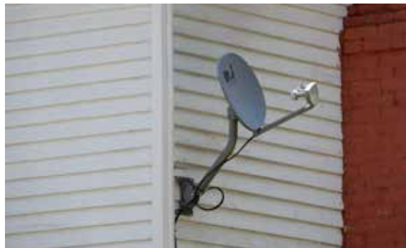
This TV dish is inappropriately mounted on the front corner of the façade of this historic dwelling and should be installed in a less prominent location.
