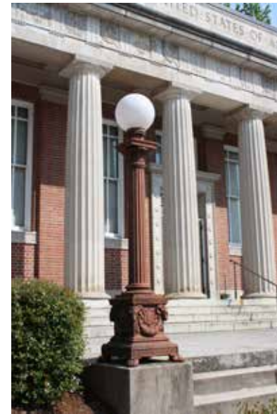
This ornate cast-metal light fixture is one of a pair & an important character-defining element to the U. S. Post Office building.
