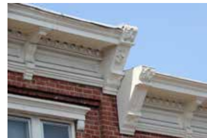
This Italianate metal cornice is highly decorated with brackets, panels and circular elements.
