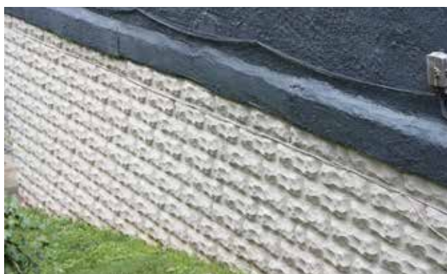
Here, artificial stone block is made from concrete formed in molds to resemble textured stone and is seen on the foundations of some early 20th c. buildings.
