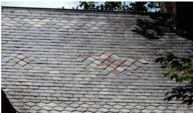
This elaborate slate roof has varied colored and shaped shingles resulting in unique decorative patterns. This example is found on a Gothic Revival-styled residence.
