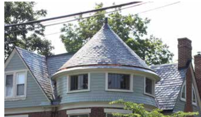
The patterned slate roof on this Queen Anne style residence is an important character-defining feature and is visually a very prominent aspect of the building's design.
