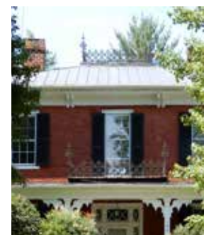
The top of this metal hipped roof is embellished with ornate metal cresting.
