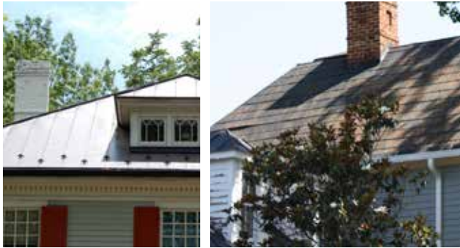
Standing-seam metal roofs are very frequently used in Lexington’s historic districts (left), while metal shingle roofs (right) are less common.
