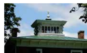
This metal hipped roof has a rare and distinctive decorative cupola capped with a finial.
