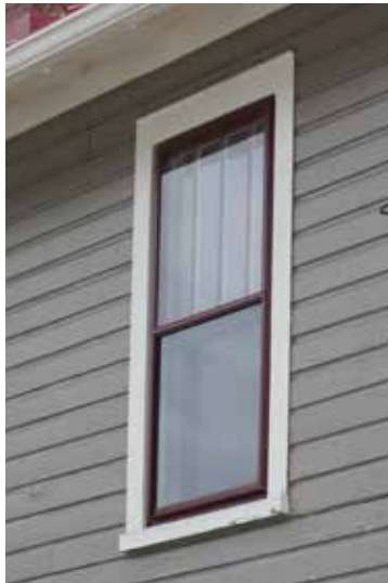
These carefully fitted storm windows match the glass window division & are painted to match other trim.
