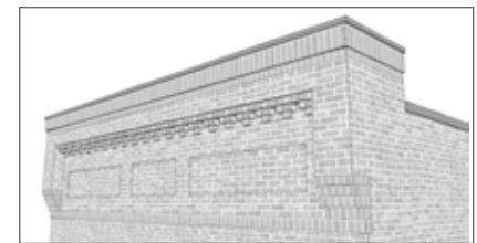
This decorative brick cornice consists of recessed panels capped by brick corbelling above. Note the soldier course at the top of the parapet wall.
