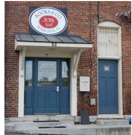
Another example of a rear entry with a similar metal shed roof. This example has a concrete base and steps added to improve entry at both doors. A wall sign above the entrance ties in with the blue color scheme.
