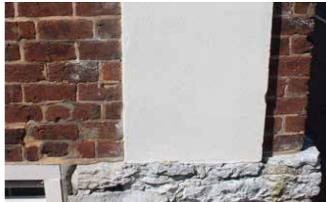
Brick is used as the primary wall material, while the brick pilaster was parged (coated with plaster) on this building.
