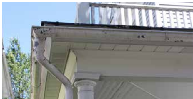
Galvanized gutters & downspouts must have the proper primer, or the paint coat will not adhere to the metal.
