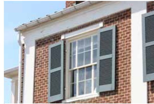
Brick with plaster pilasters and wood lintels with cornerblocks are details that help define this Greek Revival style.
