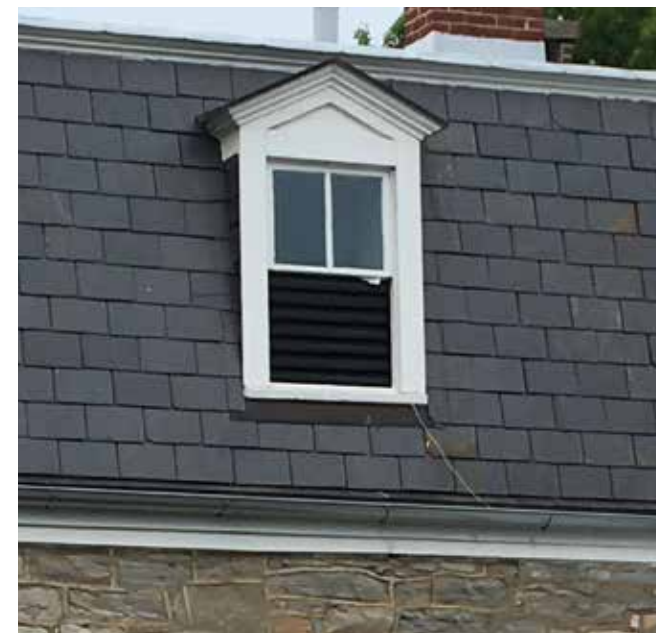
Window ventilation is an important element to install in a mothballed historic building.
