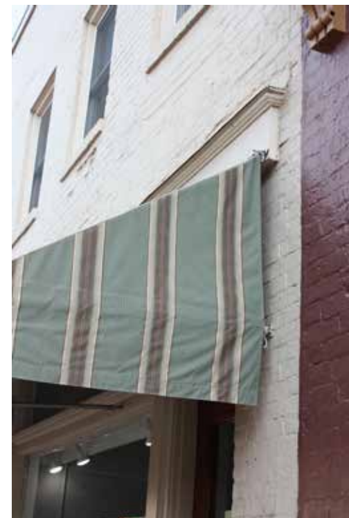
A simple metal frame with hooks on the storefront supports this non-operable awning. Attachments to brick should be made into a mortar joint, as shown here, in order to avoid damage to the brick.
