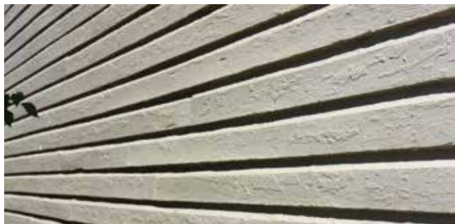
Alligatoring occurs when there are so many coats of paint on the wood that sections begin to no longer adhere to it.
