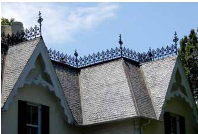
This is another Gothic Revival-styled house with a patterned slate roof consisting of alternate rows of rectangular shingles with round scalloped examples.
