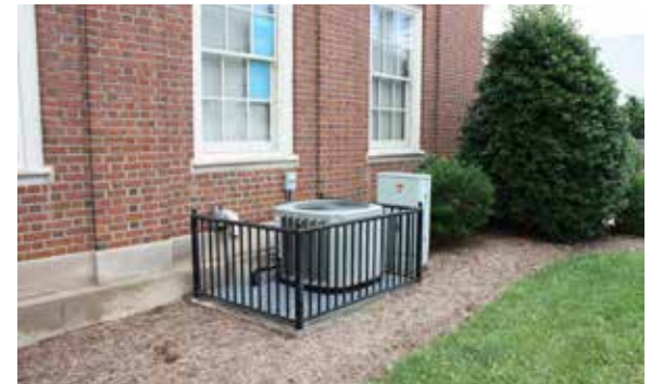
This HVAC compressor is protected by a painted metal fence but not screened because of air circulation requirements.
