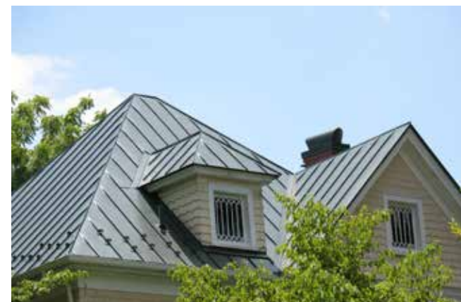
This complex metal roof is a very visible and important element in this historic house's design.
