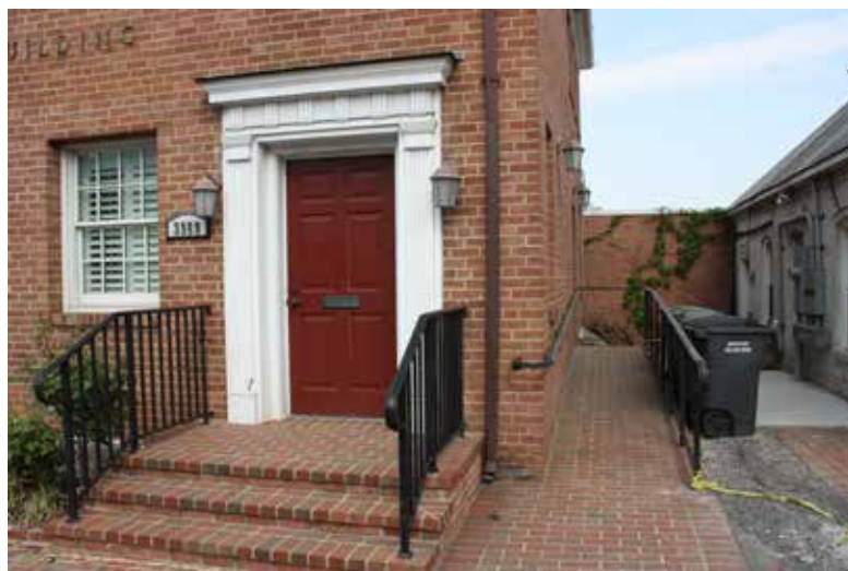
The space between these buildings allowed room for an accessibility ramp to this brick structure. The ramp was also constructed of brick to relate to the historic building.
