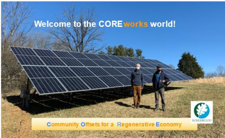
Boxerwood Solar Collector funded through CORE works.
